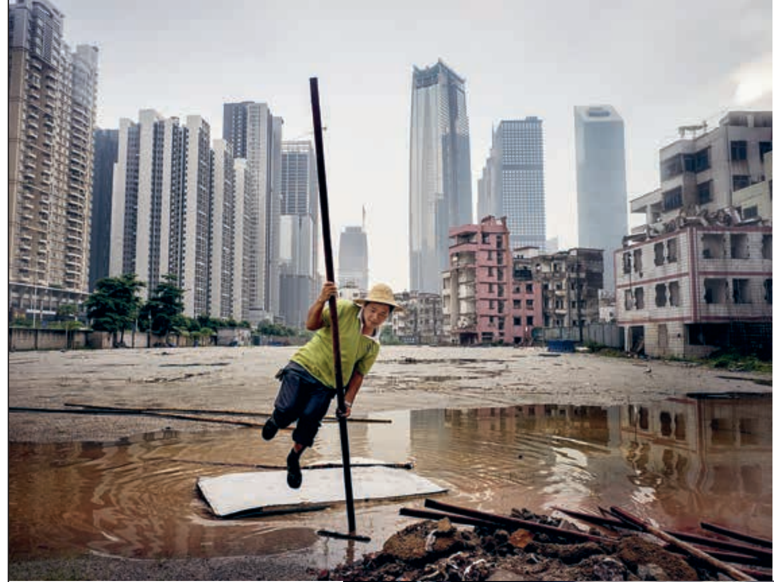
Jul 20/15. A migrant worker does an impromptu pole vault to get over a puddle while installing cables near a half-demolished urban village in Guangzhou, southern China. Photo by: @chinyin_sim @wipphoto.
